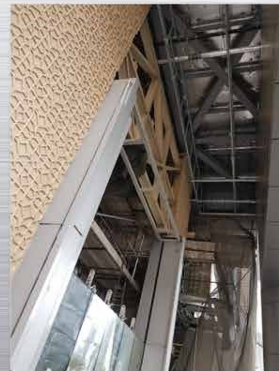
TDM ZAABEEL EXPANSION RETAIL LINK BRIDGE; INTERIOR FIT OUT. LOCATION: DUBAI MALL, DUBAI UAE CLIENT: EMAAR MAIN CONTRACTOR: QOWAT ALFAN TECHNICAL WORKS LLC
