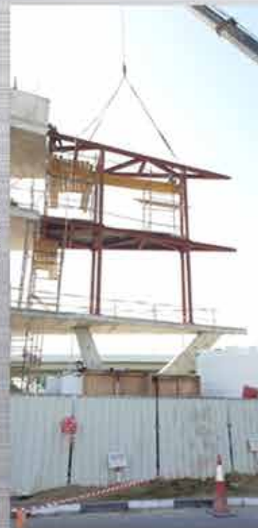
CLIENT- HASHIM CONTRACTING & GEN MAINTENANCE CO LLC PROJECT- STEEL FRAMING FOR 2 FLOORS & DECKING SHEET WITH 8 CIRCULAR STEEL COLUMN
