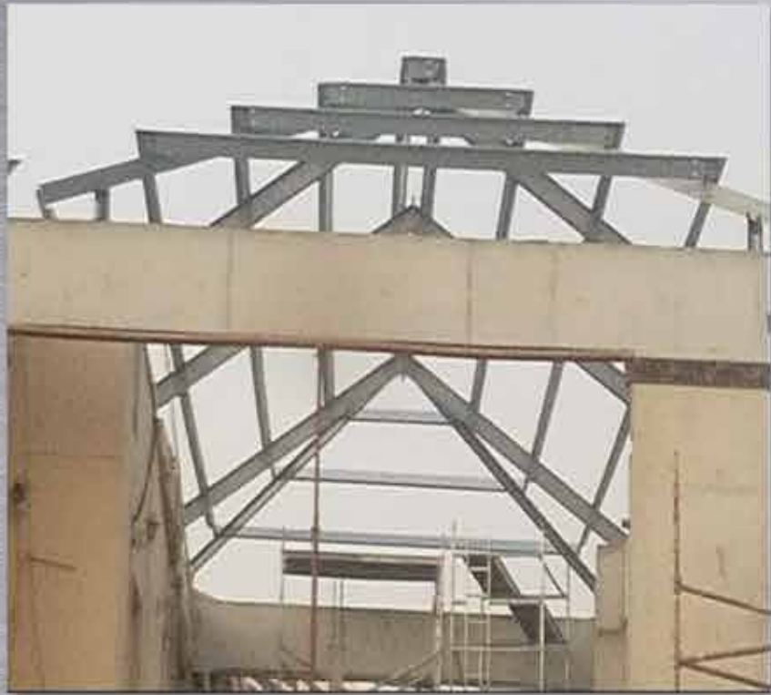
STEEL STRUCTURE FOR ROOF CANOPY LOCATION: PLOT NO. 416-1209 KHAWANEEJ DUBAI UAE CLIENT: MR. MUHAMED ARAB. CONSULTANT: AL JAWAHER ENGINEERING CONSULTANT MAIN CONTRACTOR: RASHID AL SHAMSI BUILDING CONTRACTING LLC
