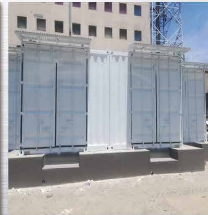
FABRICATION AND SUPPLY OF 04 NOS. INSULATED CONTAINERS FOR POWER MODULES & BATTERY BANKS FOR JAZZ DATA CENTER- PINDI STOP, KOT LAKHPAT INDUSTRIAL ESTATE ,LAHORE CLIENT: MOBILINK, PAKISTAN
