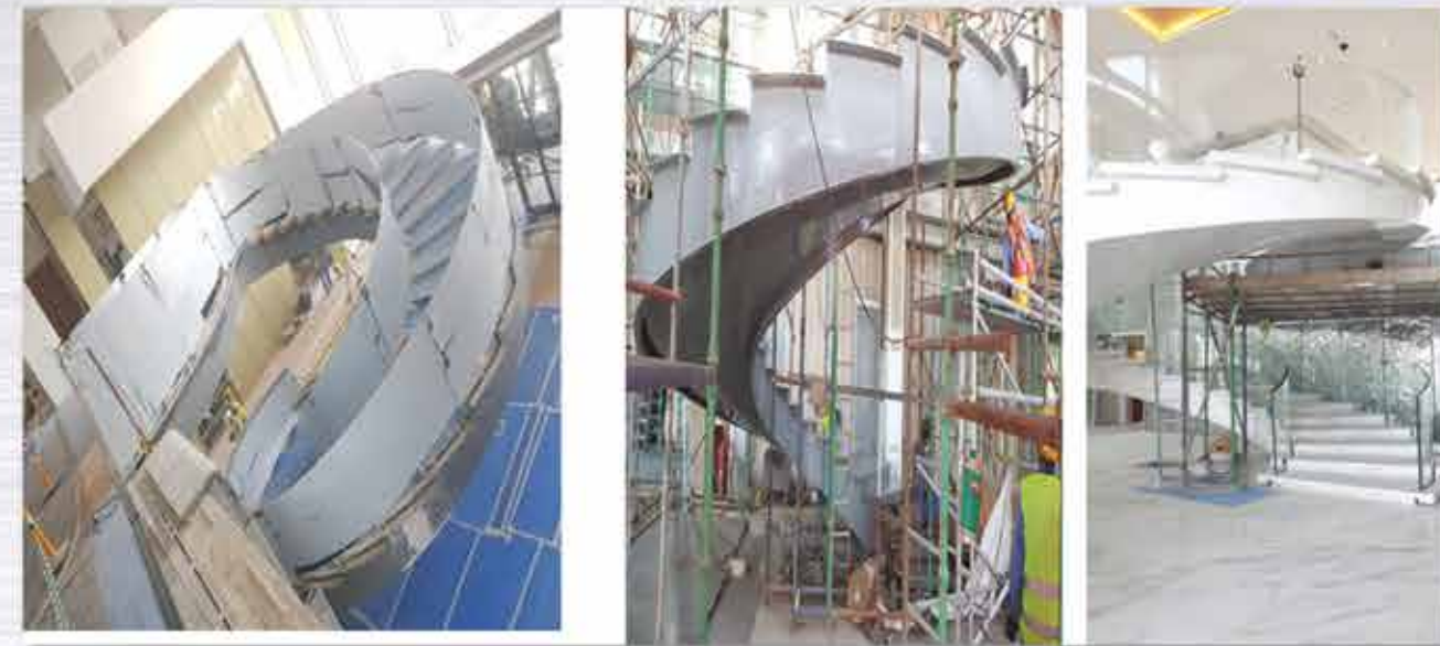
PROJECT-GRAND ENTRANCE STAIRCASE -THE ROYAL ATLANTIS RESORT AND RESIDENCES CLIENT-SANGYONG - BESIX JOINT VENTURE
