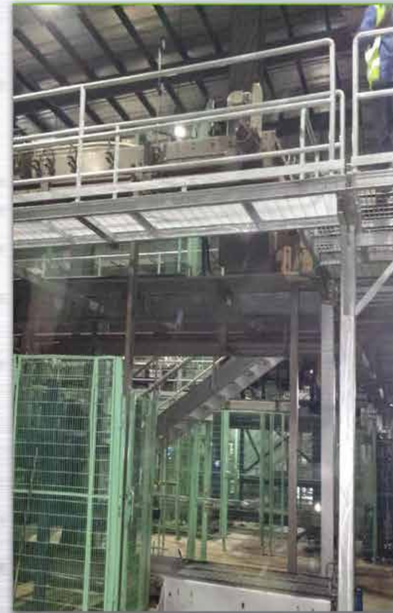
PLATFORM AND WALKWAY - AUJAN INDUSTRY
